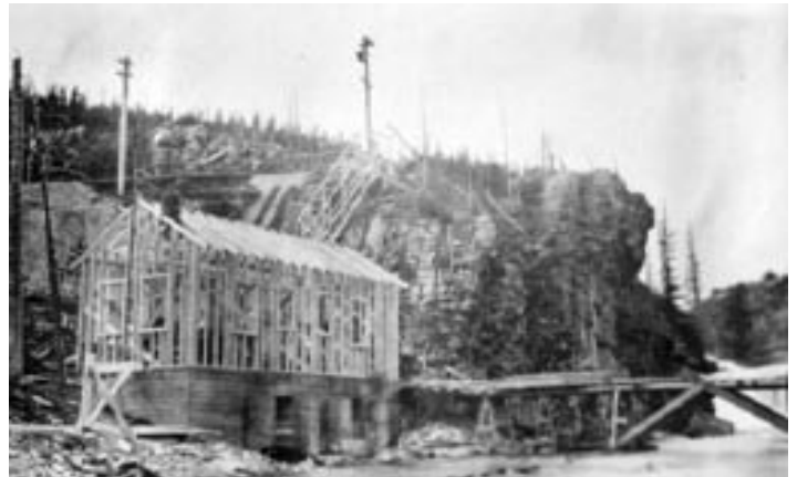
Construction of the hydroelectric power plant for Many Glacier, below Swiftcurrent Falls. (Ray Sleeper photo)
