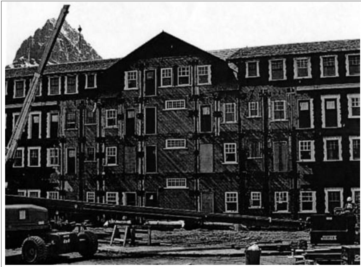
Renovations in progress at Many Glacier Hotel during Fall, 2001. Balconies and siding stripped from the main wing of the hotel have since been replaced. (Park Service photo)
